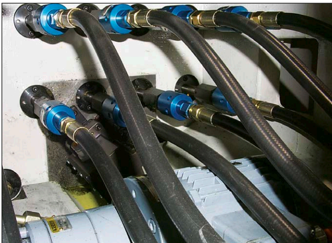
Deublin 1116 Bearing-Supported Unions on Automotive Transfer Line.
