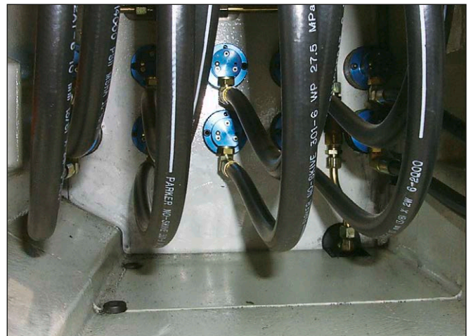
Deublin 1117 Bearingless Unions on Automotive Transfer Line.
